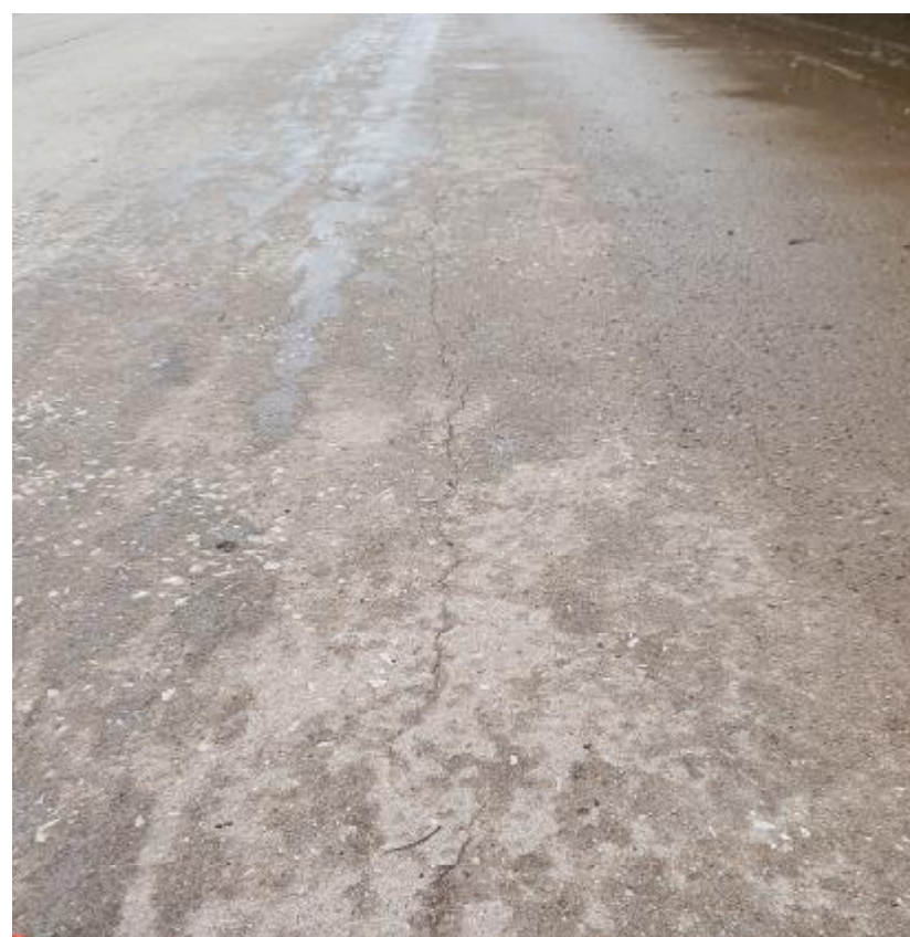
桥面铺装纵向裂缝、磨光、露骨
