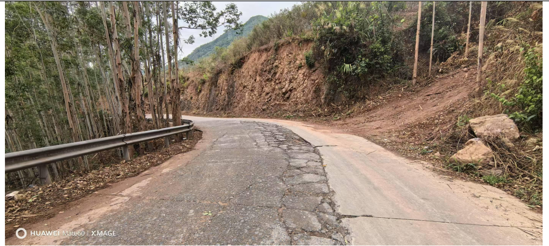
断裂、碎板、坑槽
